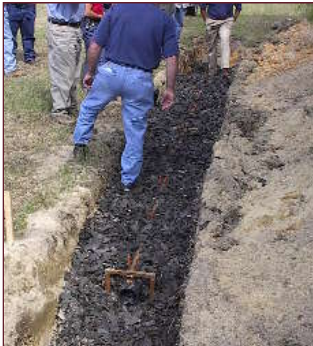
This demonstration installation of tire chips in a septic system in North Carolina featured the use of a steel brace for supporting the distribution pipe while the chips were loaded into the trench. Photo courtesy of Tim Warren.
